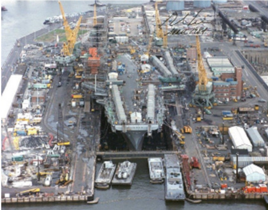
USS Forrestal (CV-59) in dock # 5 at PNSY in 1984 for its SLEP (Service Life Extension Program)
